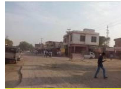
Failed Sections @ km 40.7
